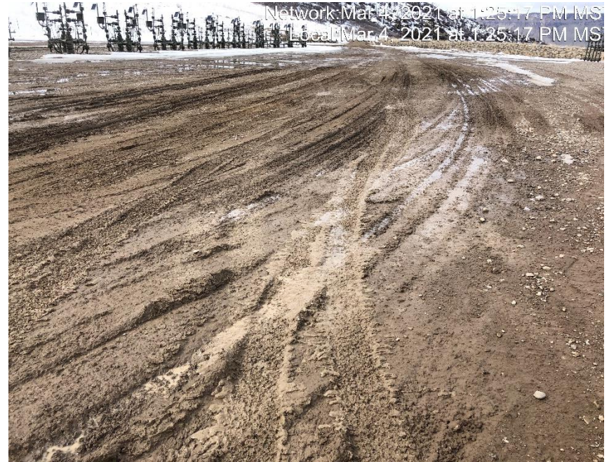
Photo #3046 Rutting present on location due to lack of stabilization.
