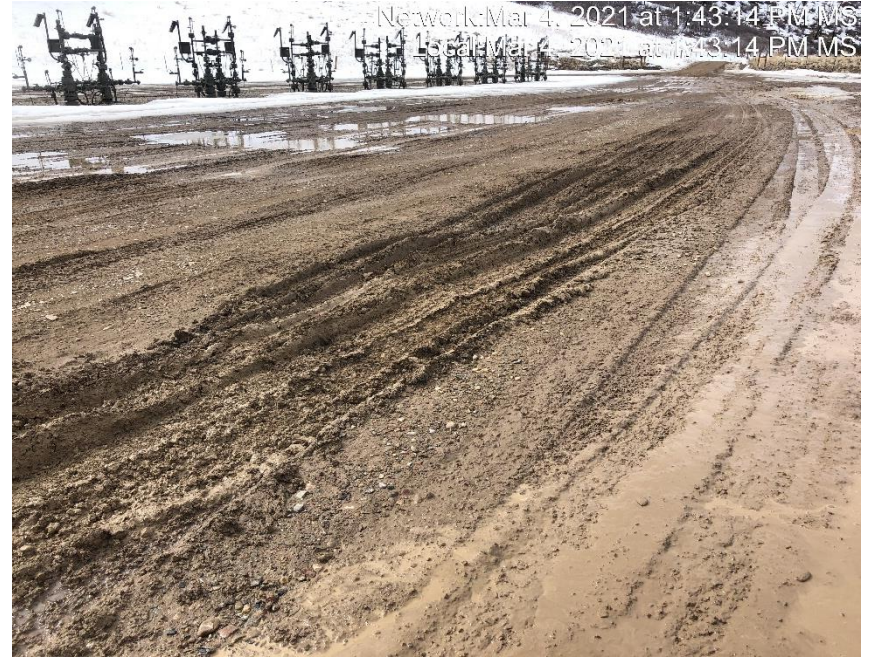
Photo #3048 Rutting present on location due to lack of stabilization.
