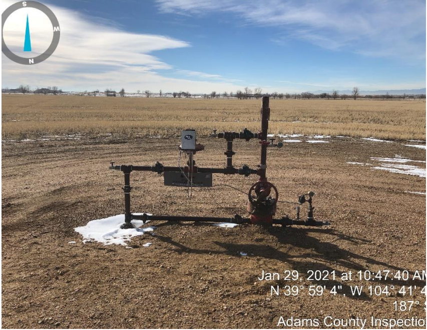
Photo #3 Well Head.
