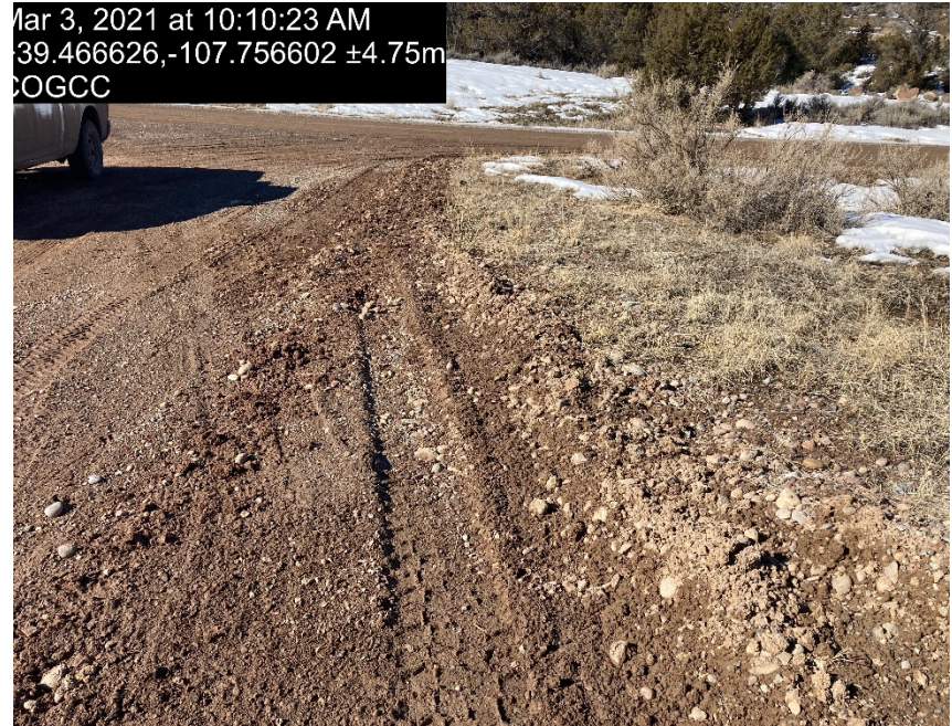
Sediment/berm plowed off of location, looking West toward entrance
