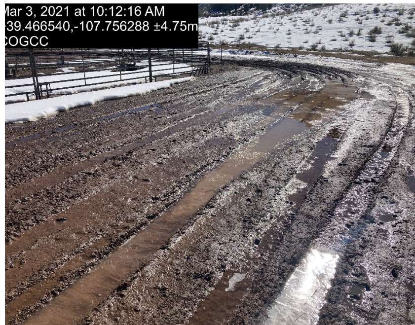
Lack of stabilization/compaction
