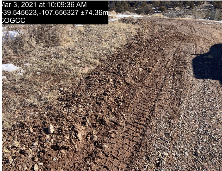
Sediment/berm plowed off of location, looking East toward location
