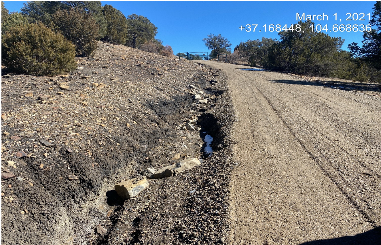
Photo 1. Facing east along the access road. There is erosion along the side of the road ascending the hill towards the gate which leads to the location.
