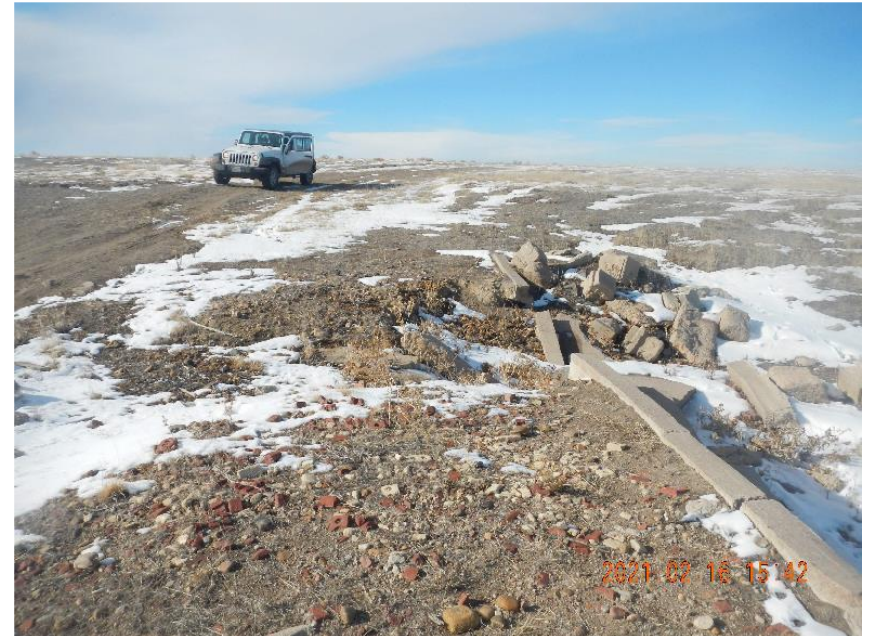
Photo 4: Access road wash out.
