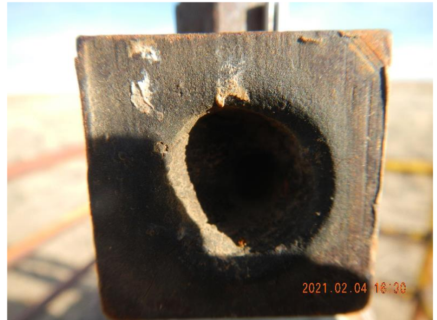
Photo 6: Valve appears to be open to atmosphere.
