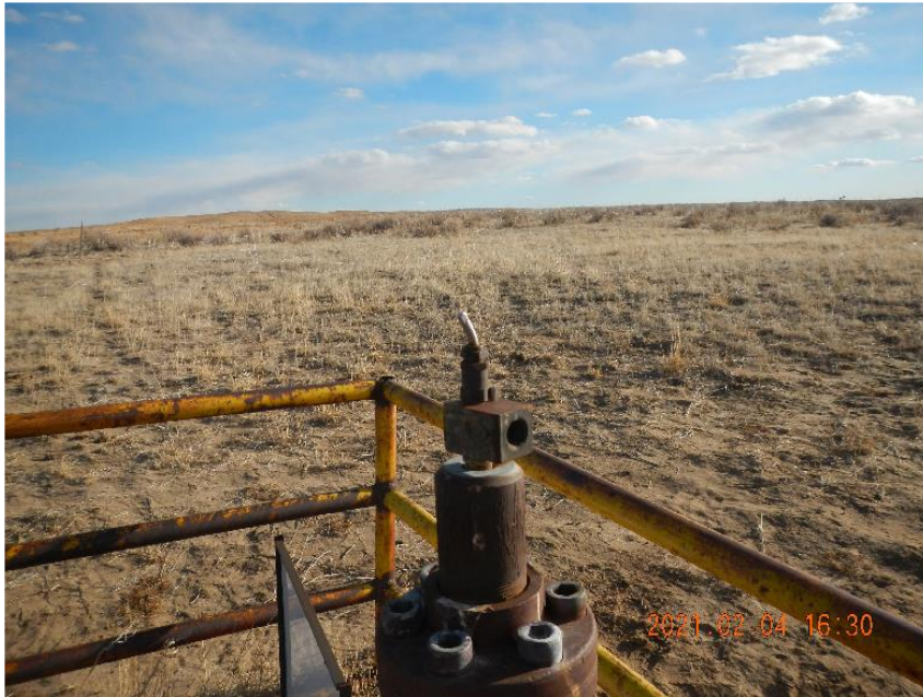
Photo 5: Broken needle valve on top of wellhead.
