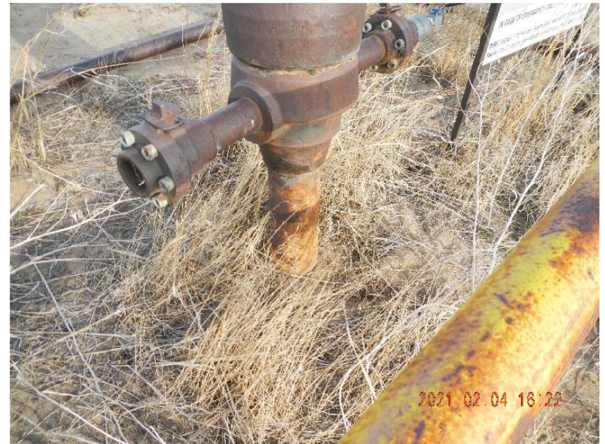
Photo 2: View of wellhead.
