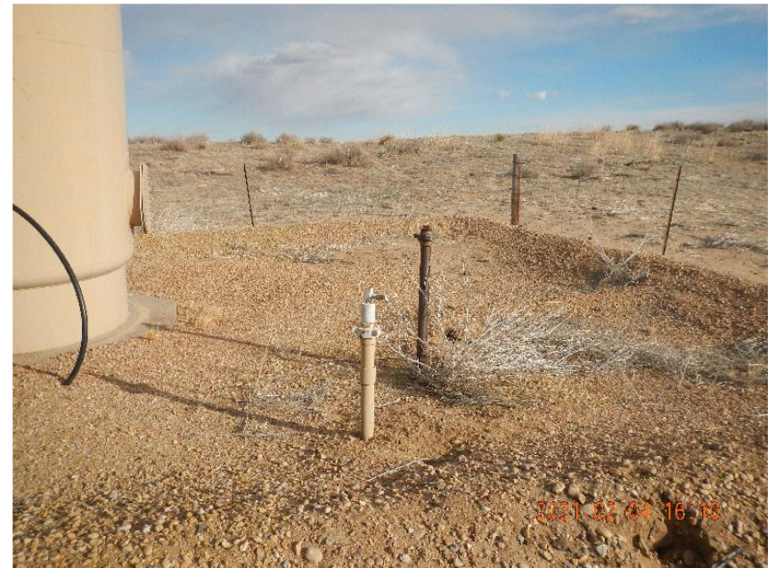
Photo 8: Plugged/capped risers at treater with no known "B" point.
