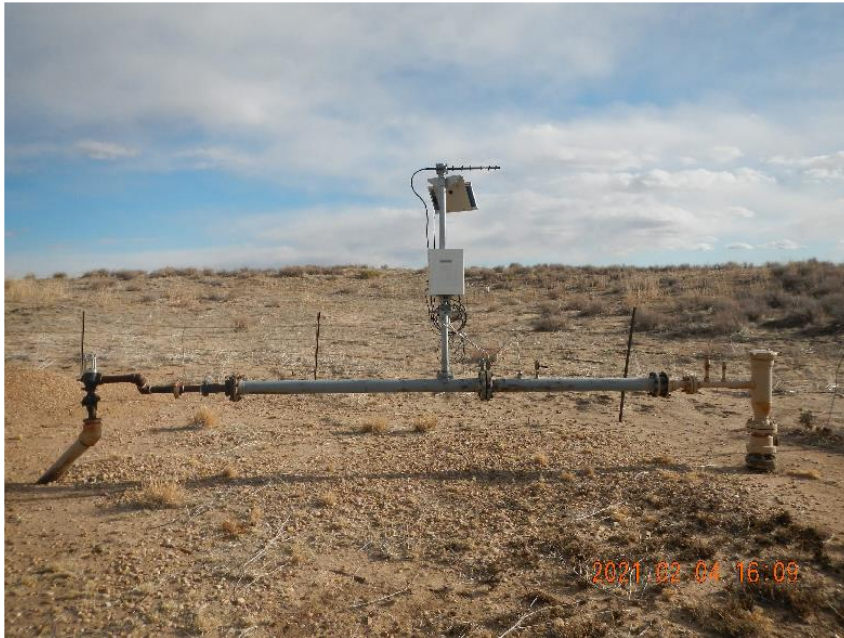
Photo 5: Gas meter run.
