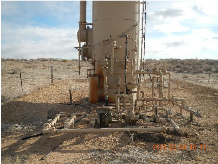
Photo 7: View of flowlines to and from treater and transfer pump.
