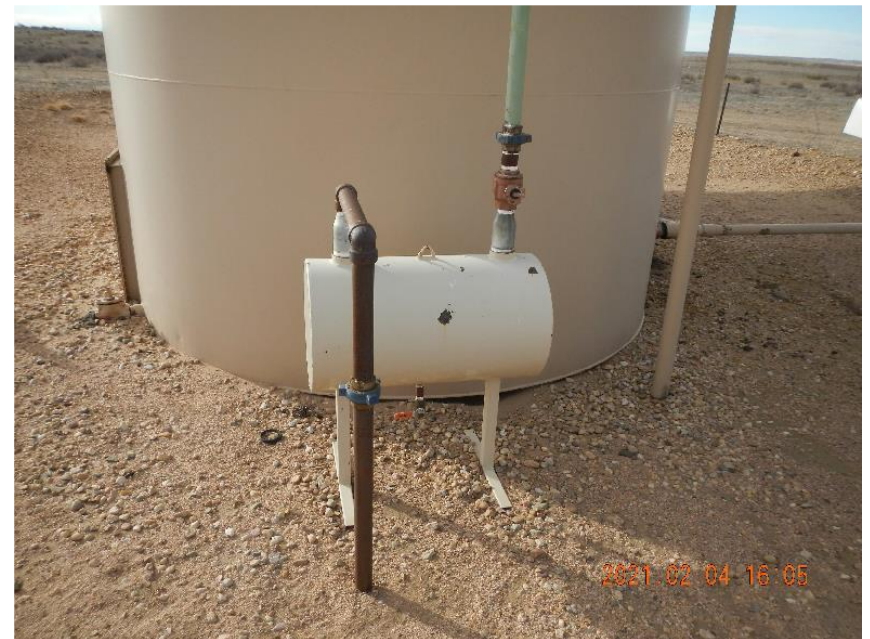
Photo 4: Knock out vessel with flowline connected.
