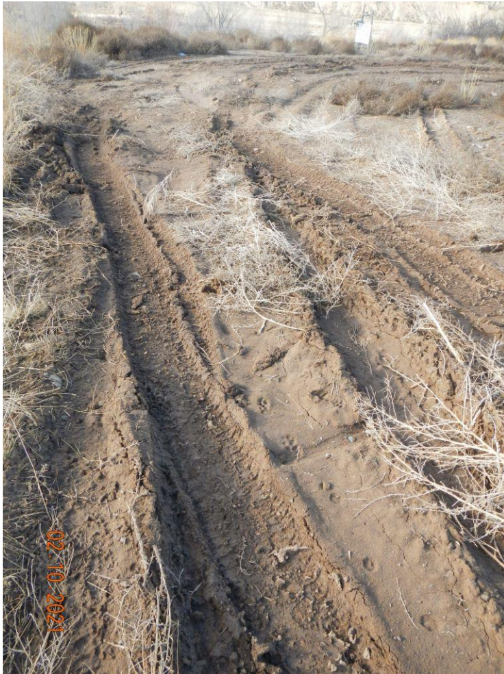
Photo#3: Close up of rutting.
