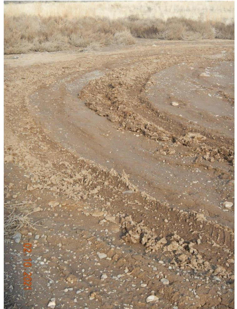
Photo#4: Close up of rutting.
