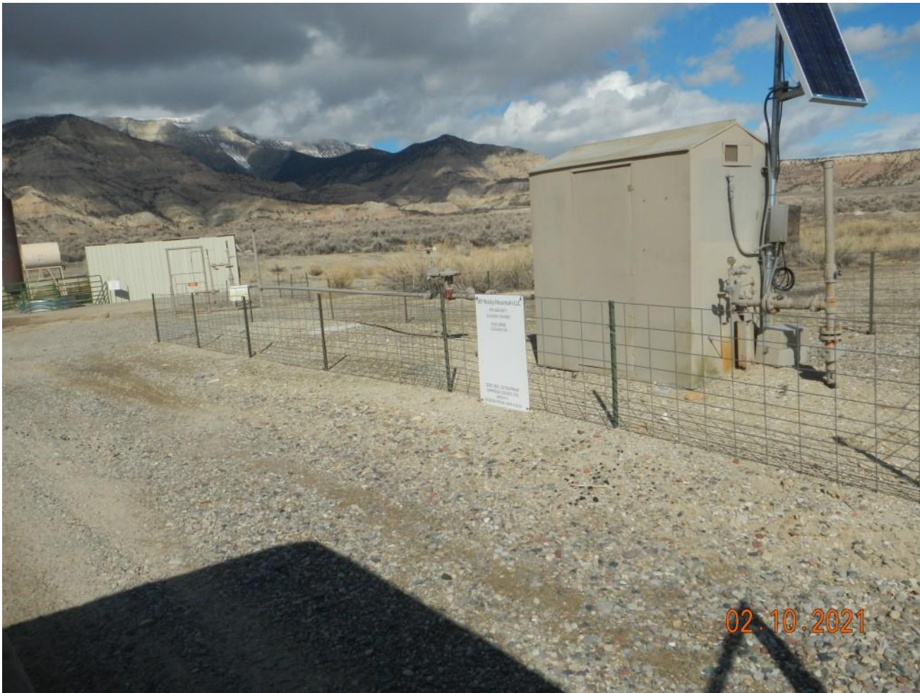
Photo#2: Overview of Location to North; Compressor Station in background.
