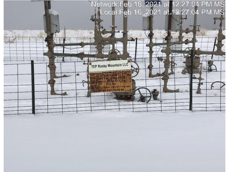
Photo #2910 Wellhead sign weathered and not legible.
