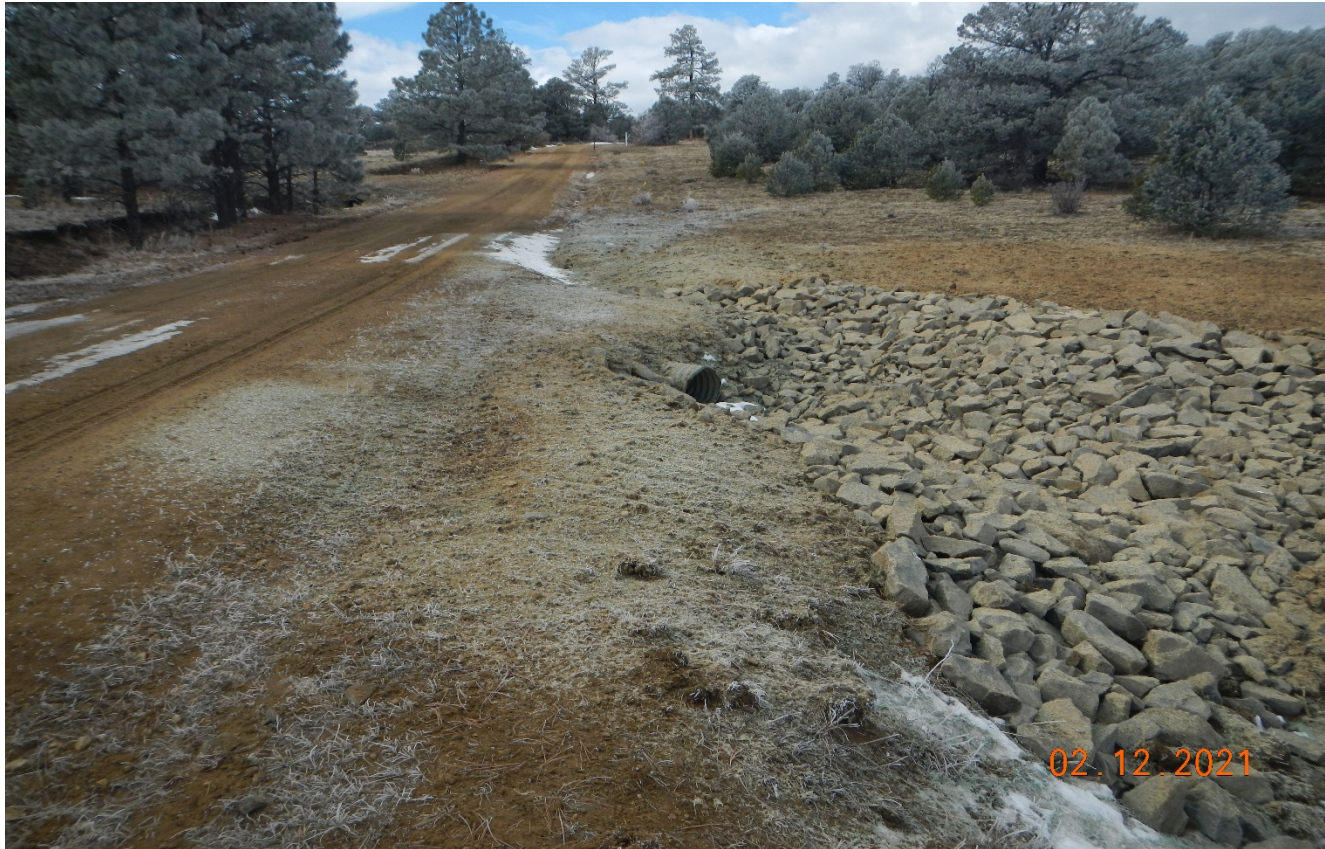
Photo 1. Facing west along the access road. Outlet protection was installed at the culvert. Rock rip/rap is installed where gully erosion was identified.
