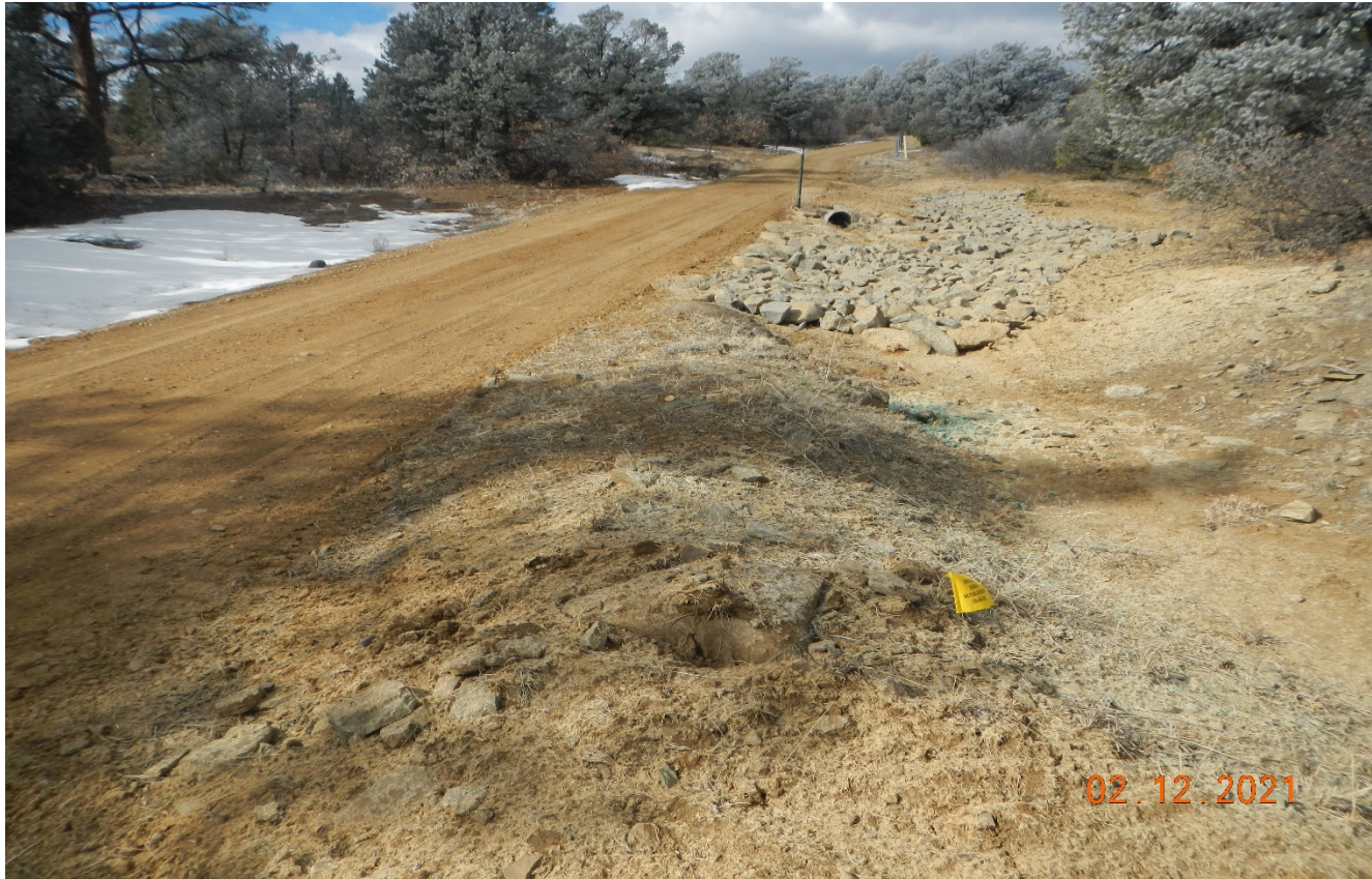
Photo 2. Facing west along the access road. Outlet protection was installed at the culvert.
