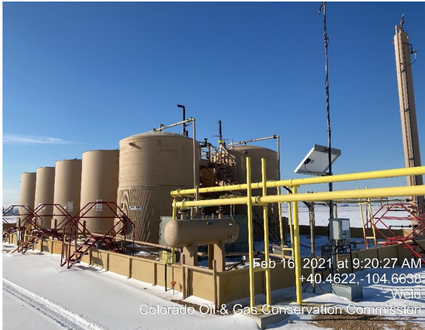
Photo #3 Tank Battery
