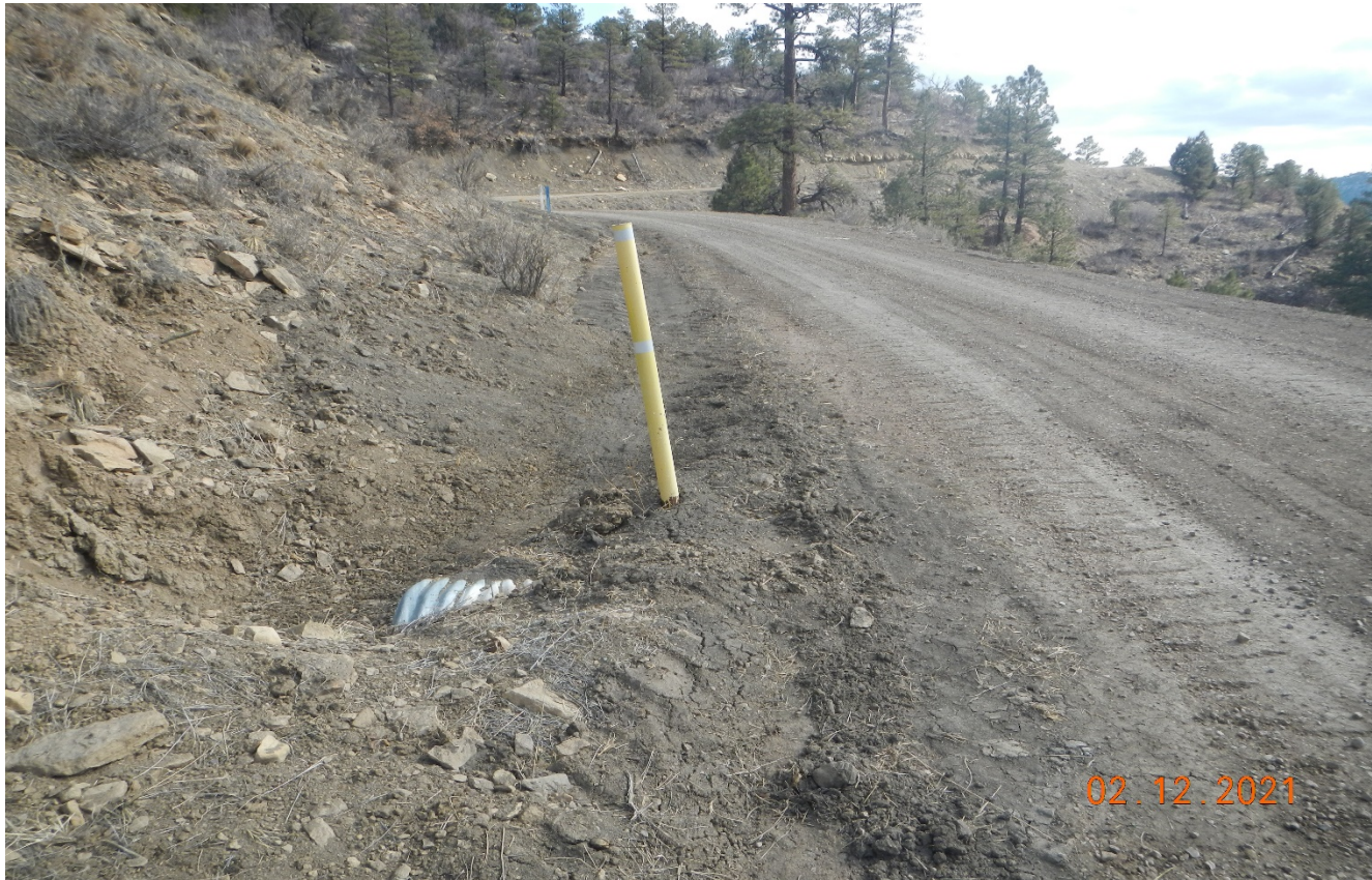
Photo 1. Facing southeast along the access road. Culverts have been maintained and cleaned out. The road has been regraded.
