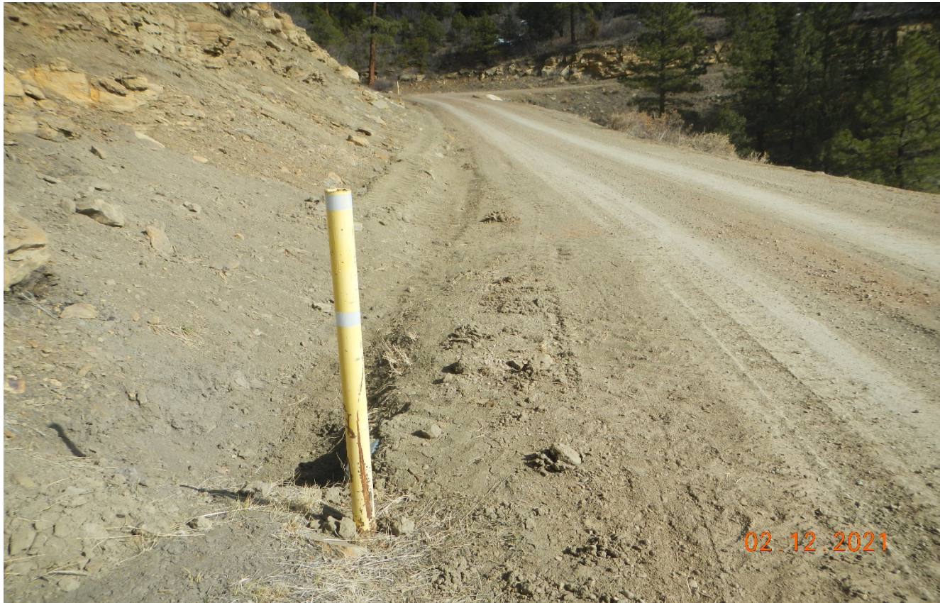
Photo 2. Facing east along the access road. Culverts have been maintained and cleaned out. The road has been regraded.
