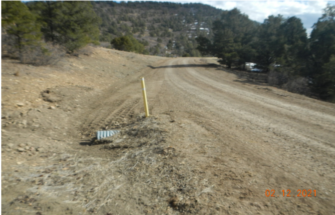
Photo 3. Facing southeast along the access road. Culverts have been maintained and cleaned out. The road has been regraded.
