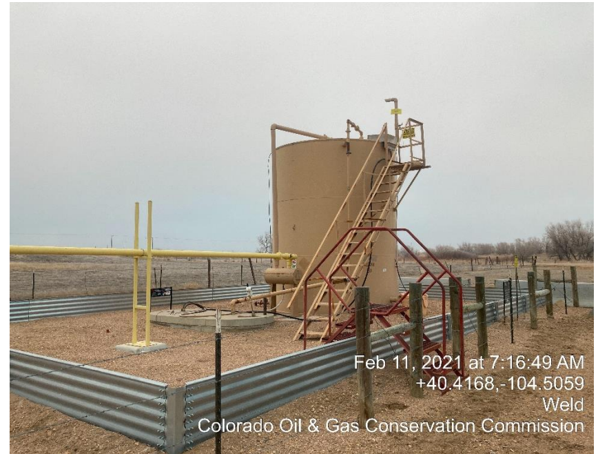
Photo #2 Tank Battery
