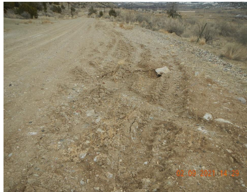
Ground subsidence where polyline is buried across access road.
