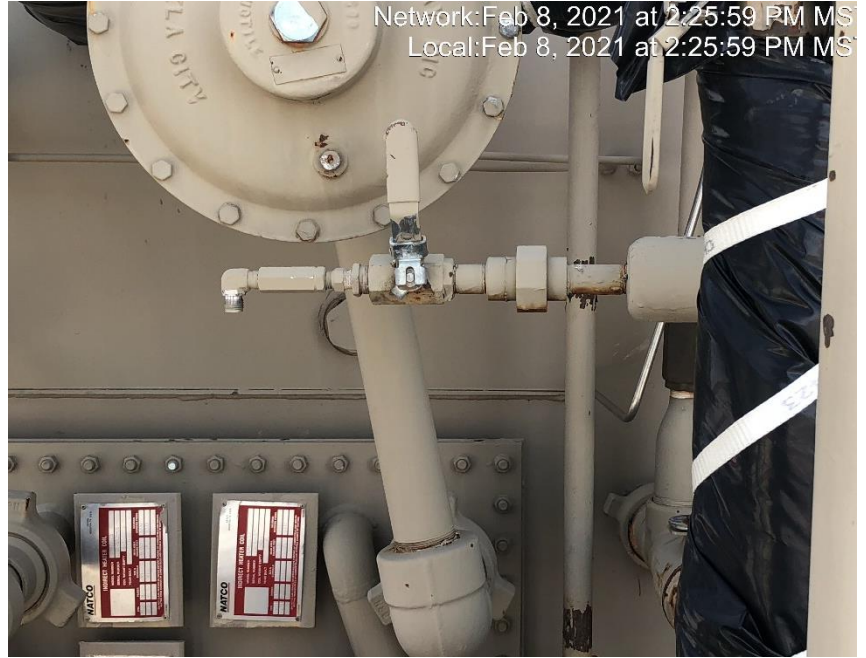
Photo #2850 3/8 stainless steel fittings.
