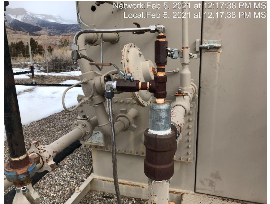
Photo #2829 3/8 stainless steel line that is connected to sales line of the separator
