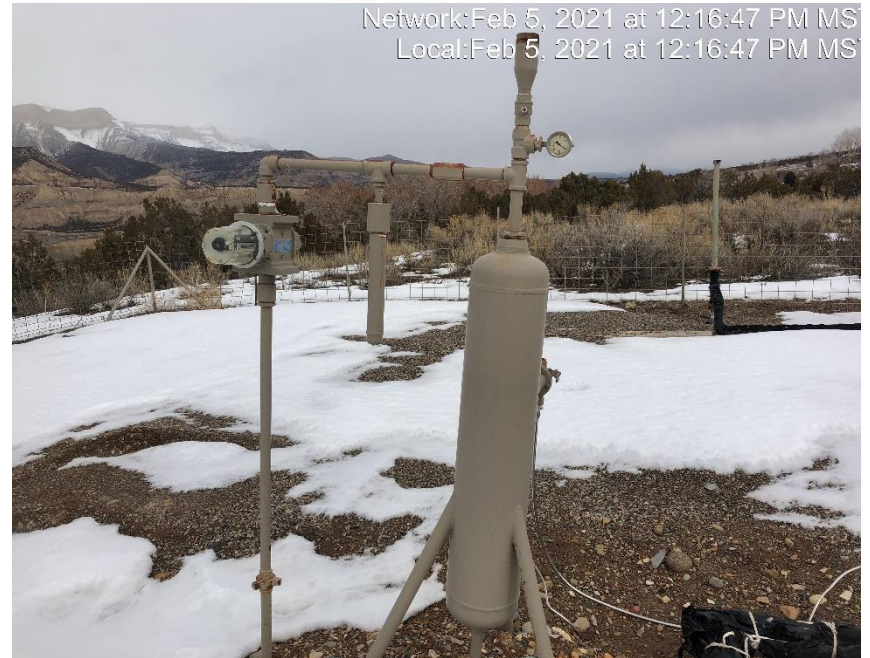
Photo #2827 knock out bottle and a domestic gas meter
