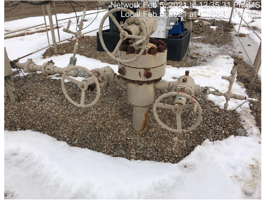
Photo #2830 Bradenhead valves are not accessible.
