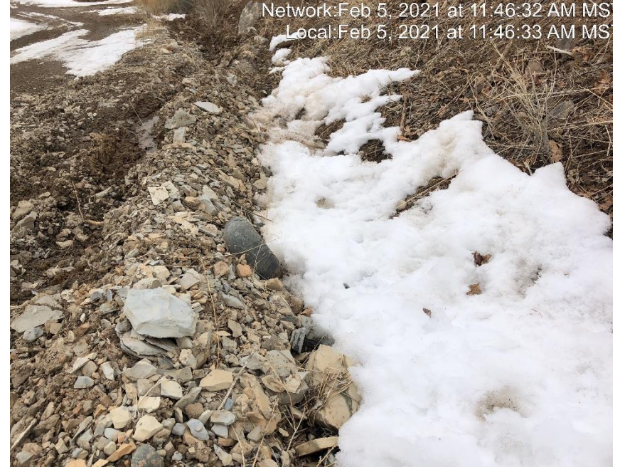
Photo #2823 Ditch has been diverted due to rutting.
