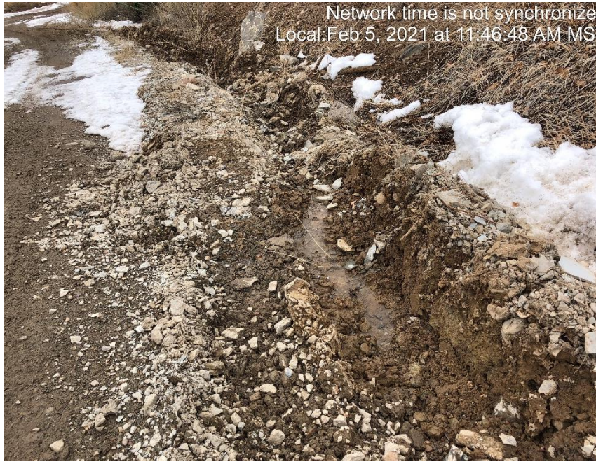
Photo #2824 Ditch has been diverted due to rutting.
