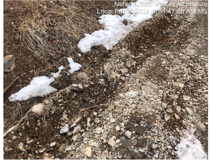
Photo #2825 Ditch has been diverted due to rutting.
