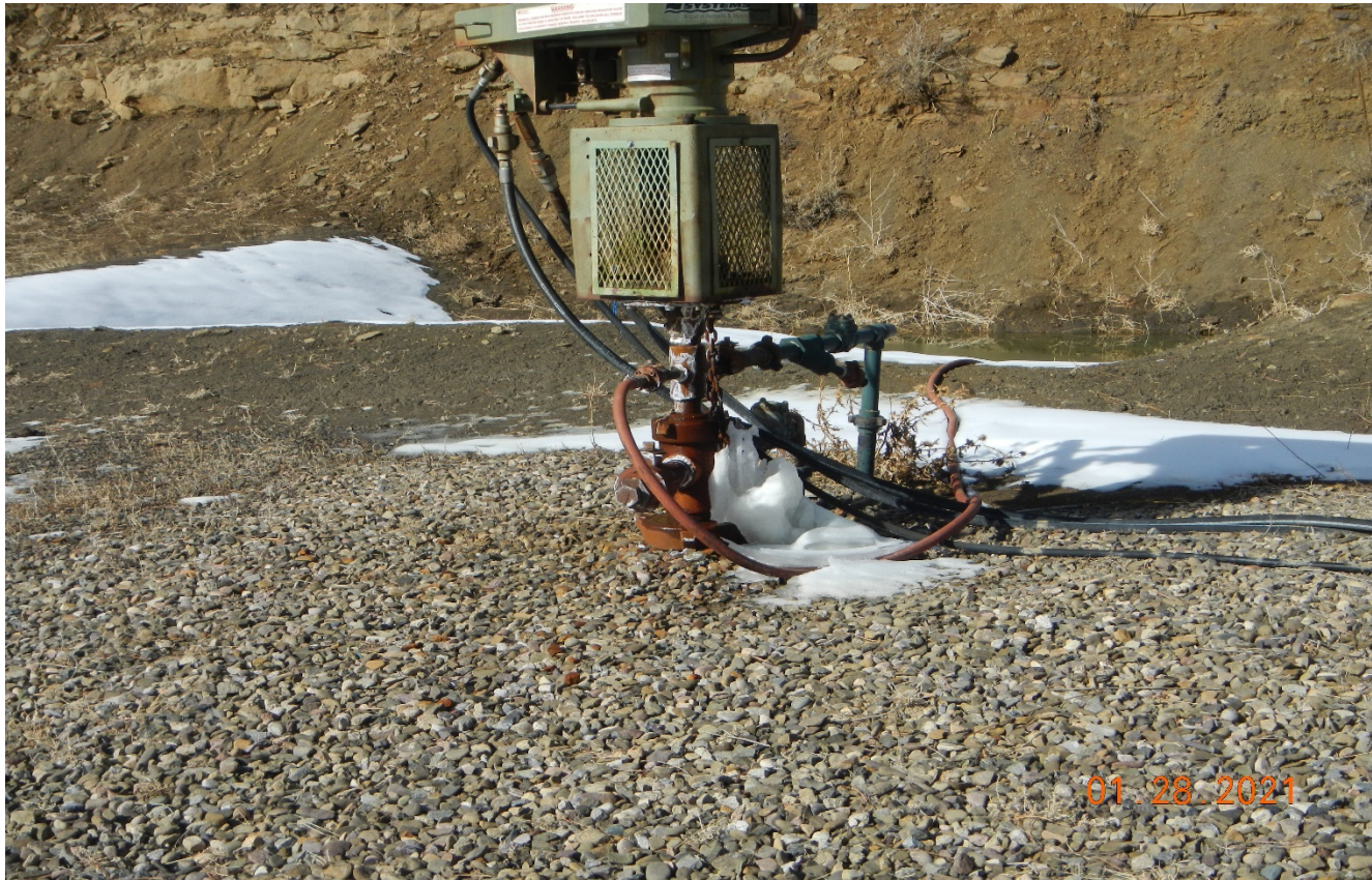
Photo 2. There is a dripping water leak at the wellhead.
