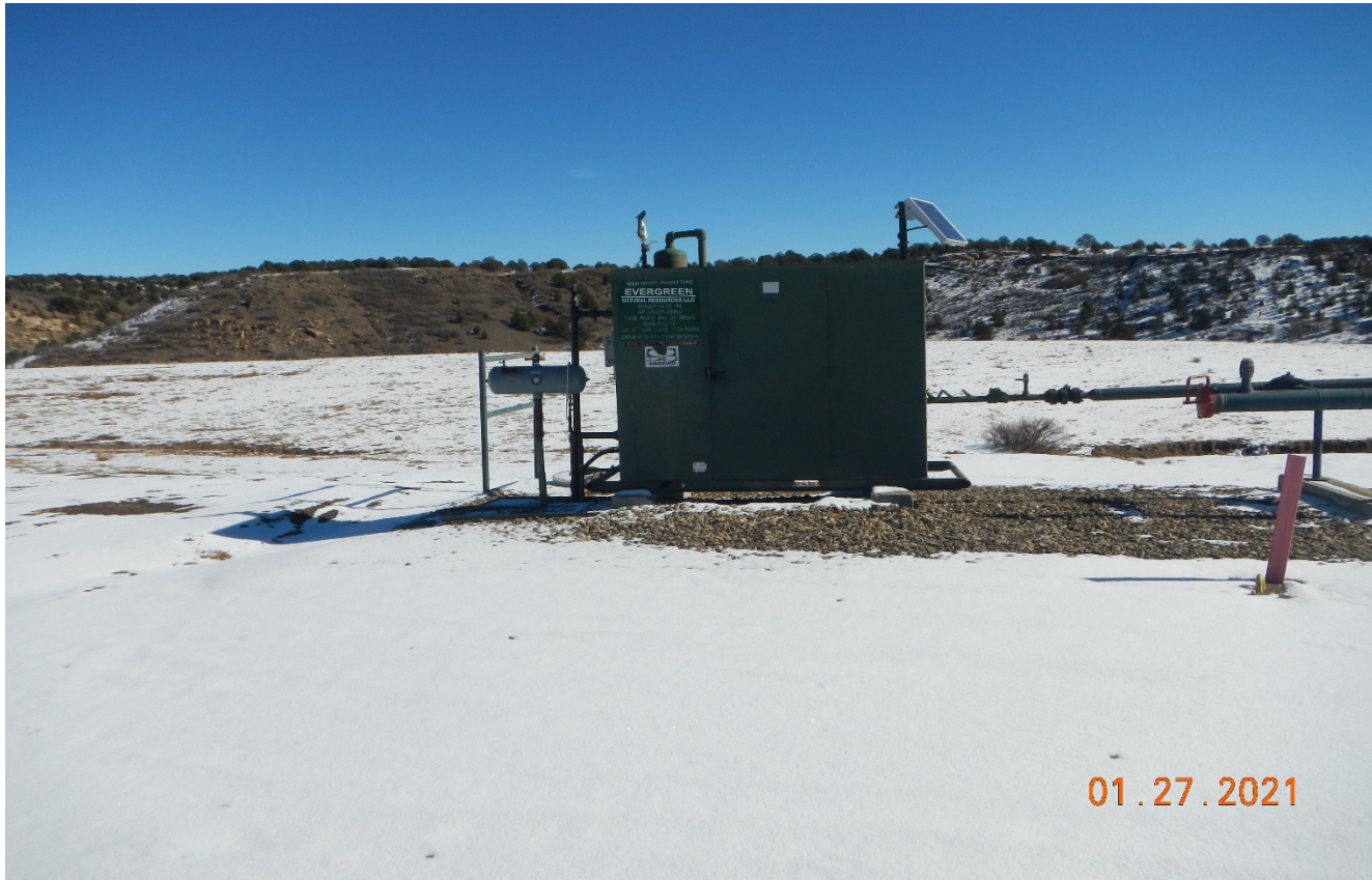
Photo 3. Well sign is posted at meter shed.
