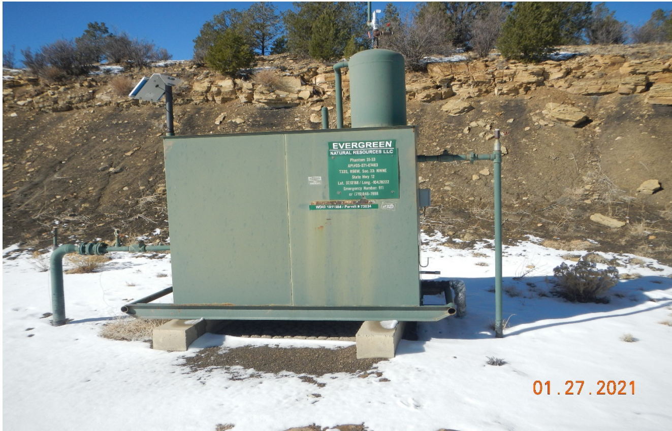
Photo 2. Well sign is posted at meter shed.
