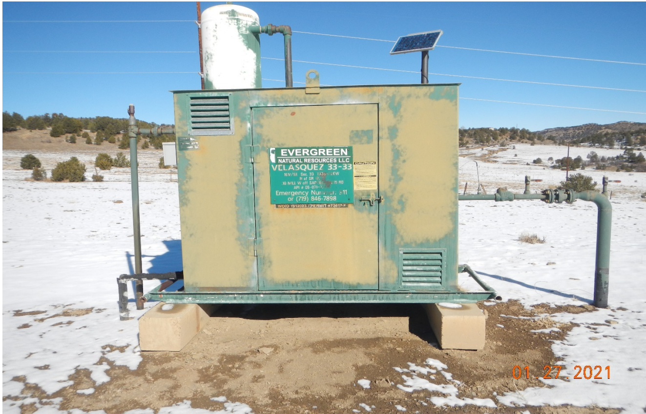
Photo 2. Well sign is posted at meter shed.
