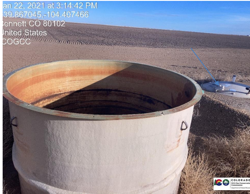
Pic 3 tank with no netting, top next to tank on ground
