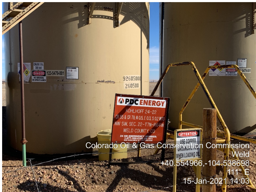
Photo #3 Kohlhoff 24-22 Battery site Inactive | Shut-down Battery sign
