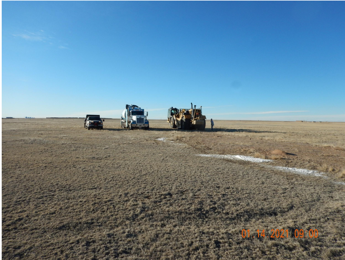
Photo 1. Photo taken from the southern access road, facing South. Photo illustrates Operator field crew commencing final reclamation activities.
