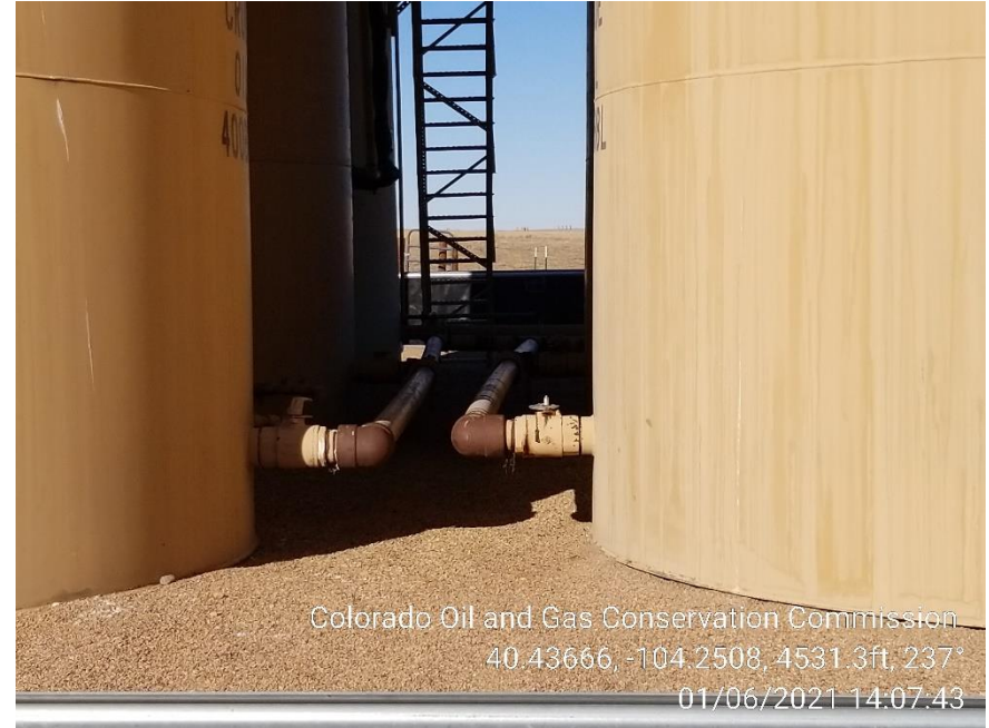
Photo 6 – Stained Soil at Loadline has been cleaned up
