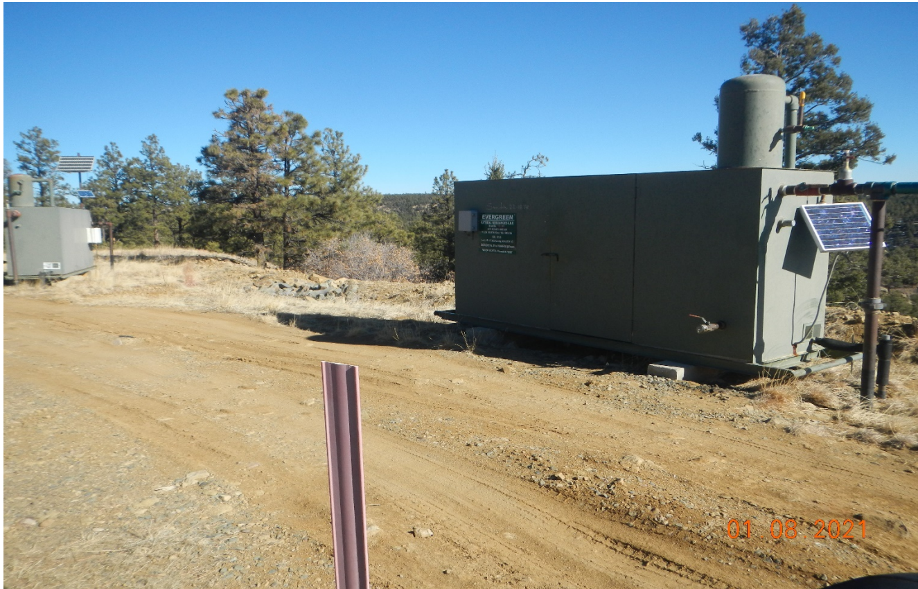
Photo 4. Well sign posted at meter shed.
