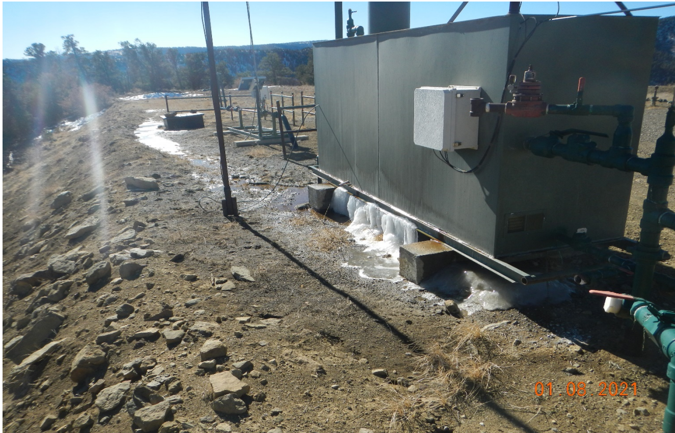
Photo 2. There is a waster leak coming from the meter shed.
