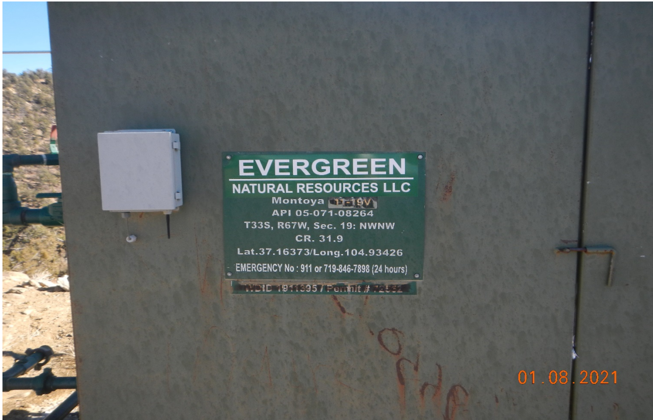
Photo 1. Well sign posted at meter shed.
