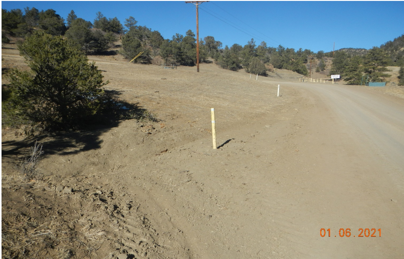
Photo 1. Facing northwest along the main access road. The culvert along the access road has been cleaned out and maintained.
