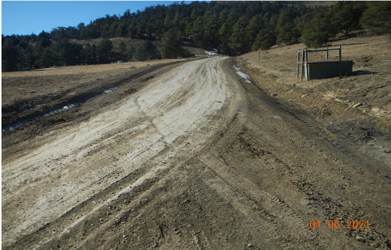
Photo 2. Facing southwest along the access road ascending the hillside. The road has been regraded.
