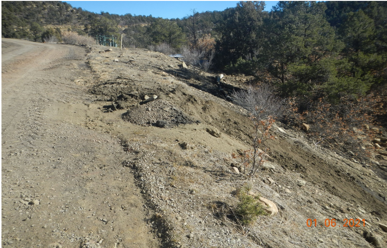
Photo 3. The erosion off the fill slope of the road has been filled in. This area will need to be seeded and stabilized.
