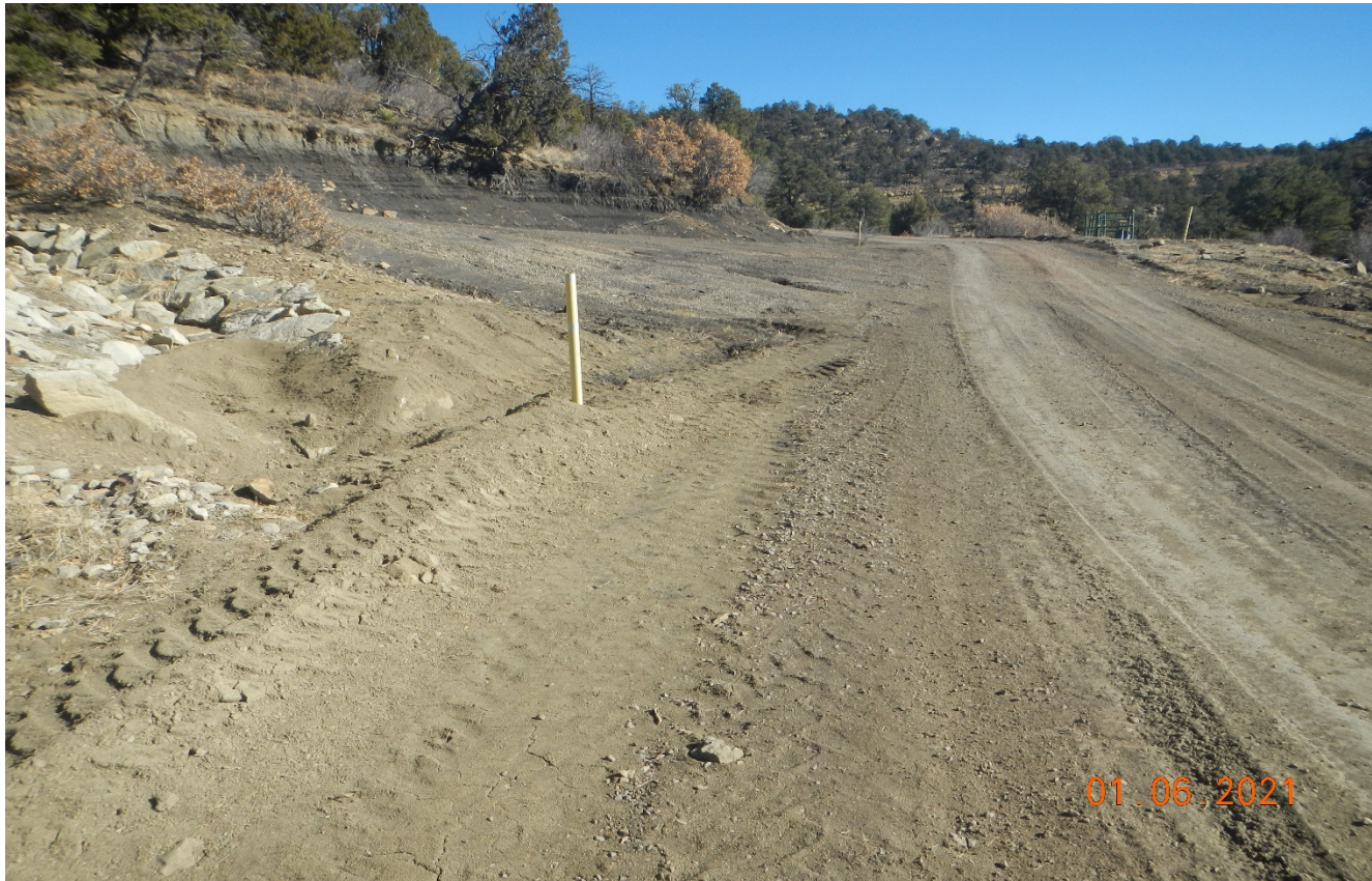
Photo 2. The culvert along the access road has been cleaned out and maintained.
