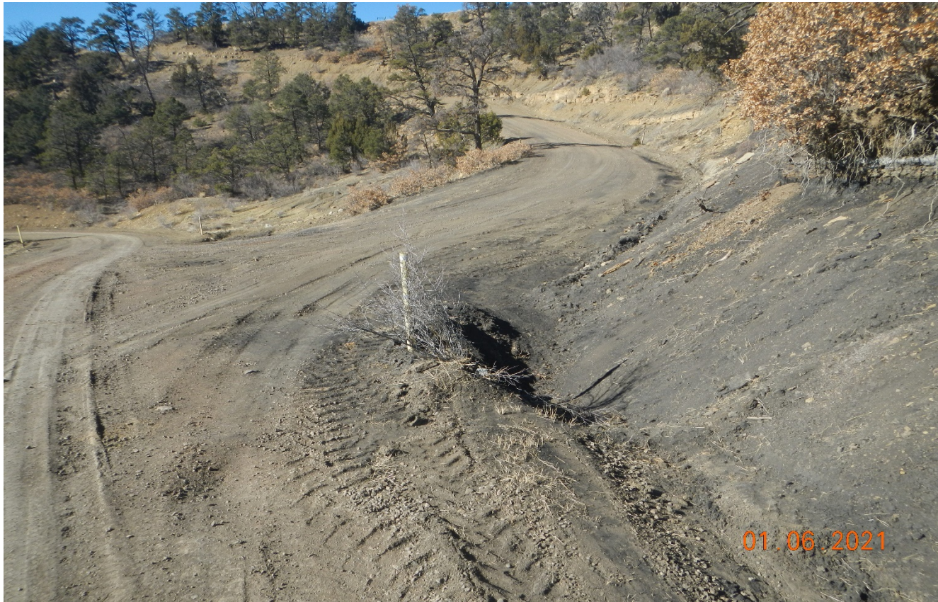
Photo 4. Facing northeast toward the access road. Stormwater The culvert has been cleaned out and diversion toward the culvert repaired.
