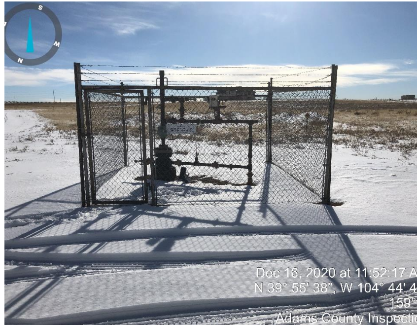
Photo #1 Well Head.
