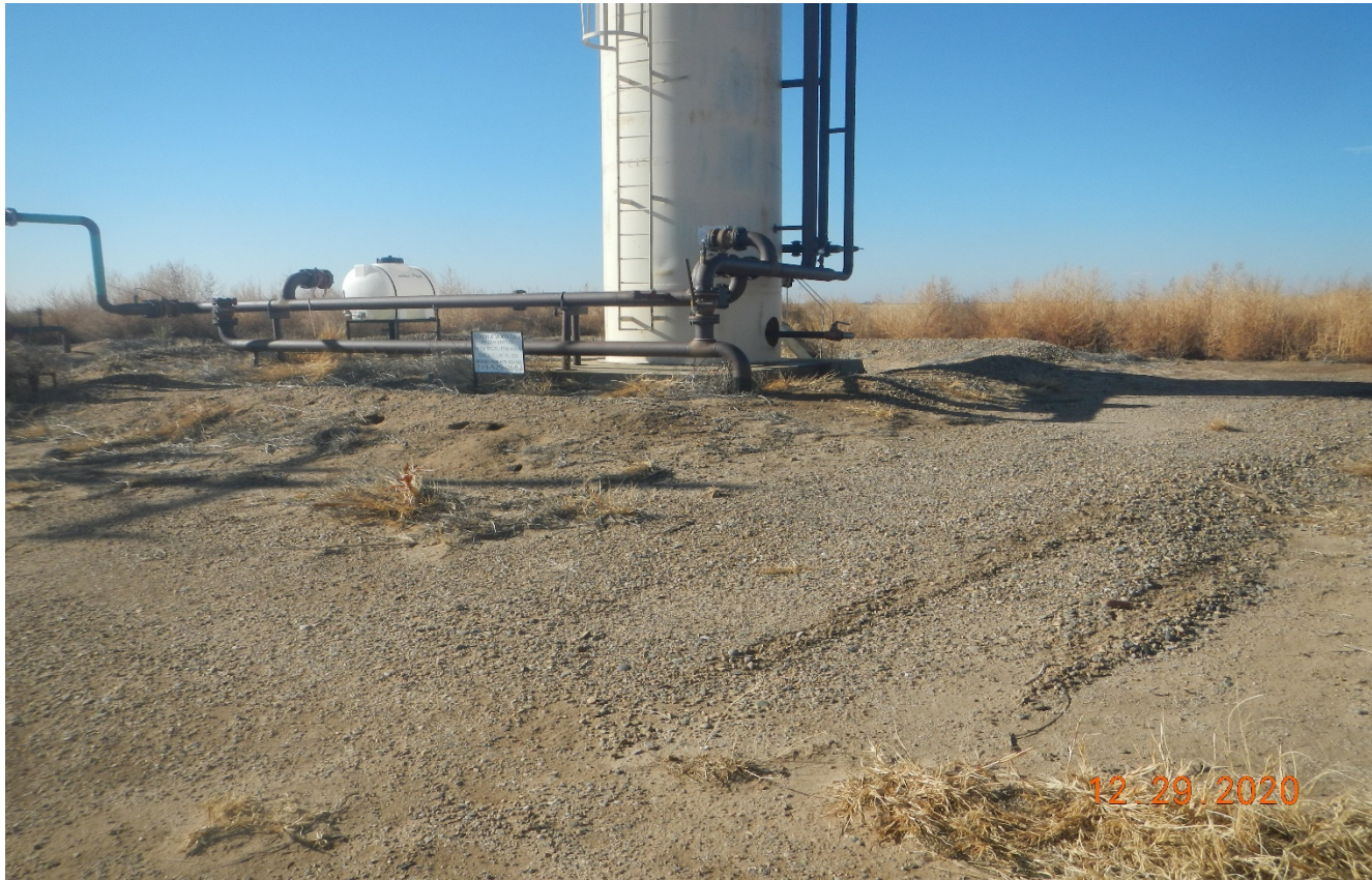
Photo 7. Facing toward the southwest side. The berm around the tank vessel is inadequate in size and has animal burrows in it.
