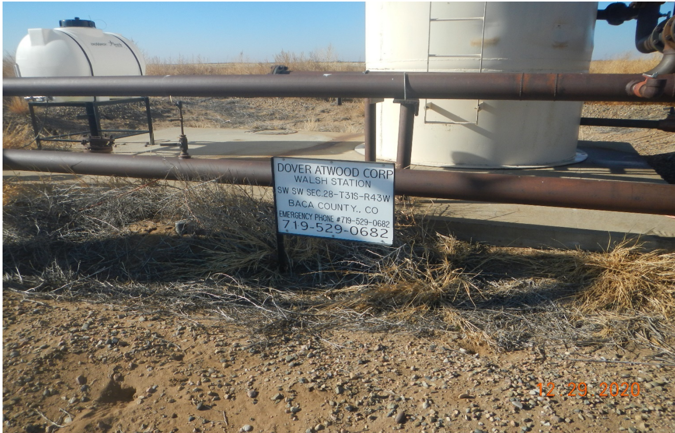
Photo 8. The facility sign is posted but contains incomplete and inaccurate information.
