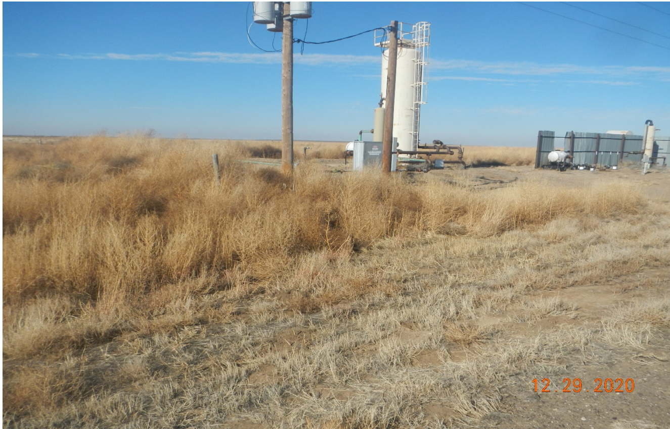
Photo 10. Facing northwest toward the location. The perimeter of the location consists of tall weeds (Kochia) debris which is a fire hazard. The weeds around the perimeter of the location need to be cut and removed.
