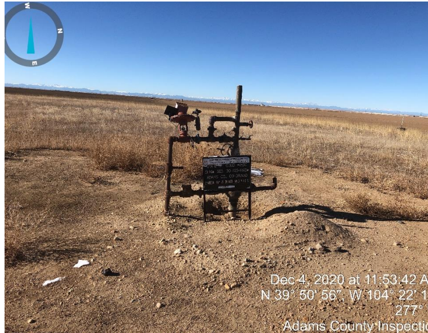
Photo #3 Well Head.
