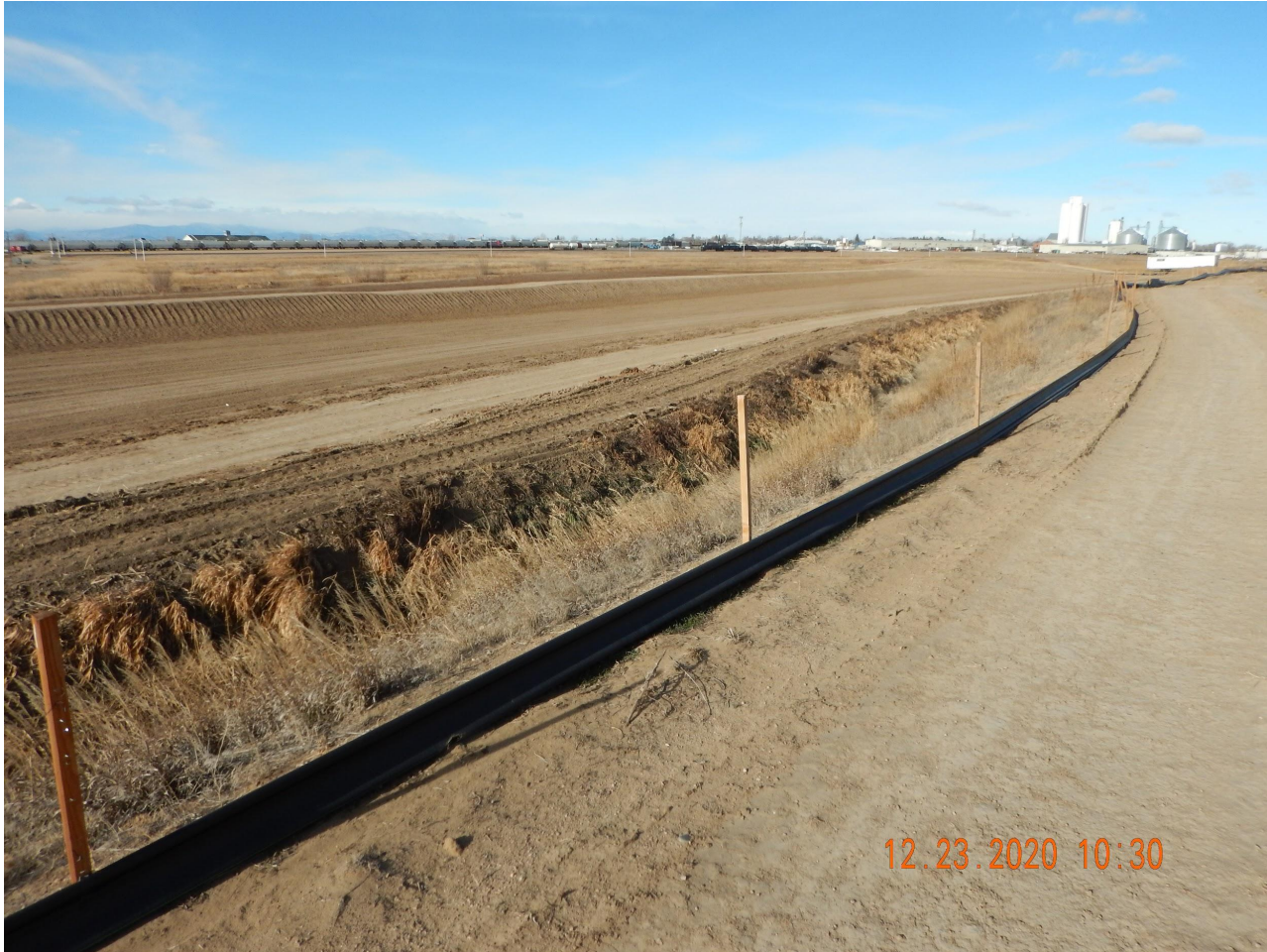
Photo 4. Photo taken from the well/tank battery location, facing Northwest. See comments under Photo 1. Photo illustrates the retention area BMP for the development.
