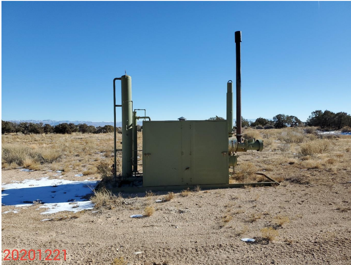
Photo 4: Photo shows separator equipment remaining on the Location.
