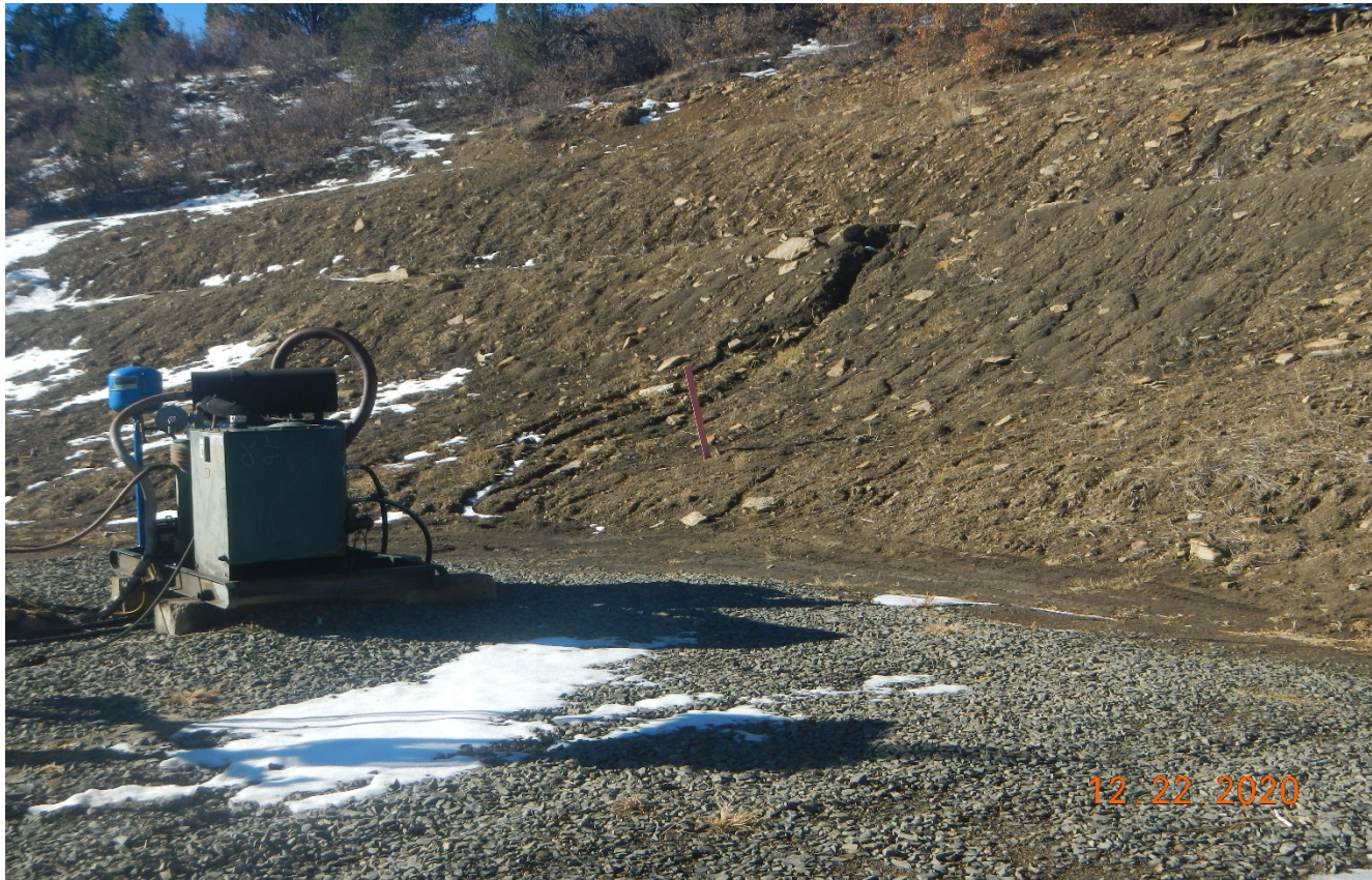
Photo 3. There is an erosion channel at the cut slope which needs to be repaired.
