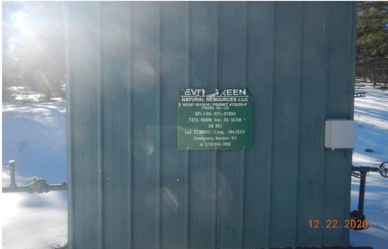
Photo 3. The operator name on sign is peeling off and will need to be replaced.
