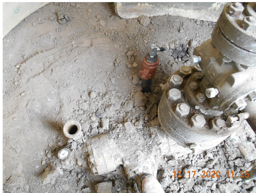
Wellhead inside housing with bradenhead valve plumbed to surface. CA completed.
