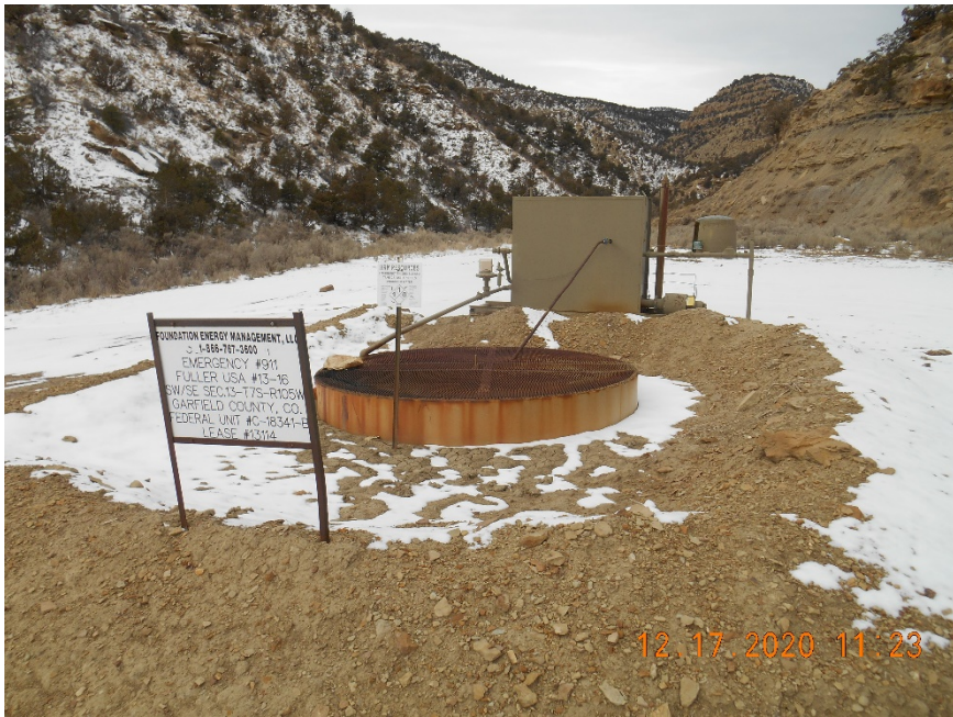
Separator and blowdown tank
