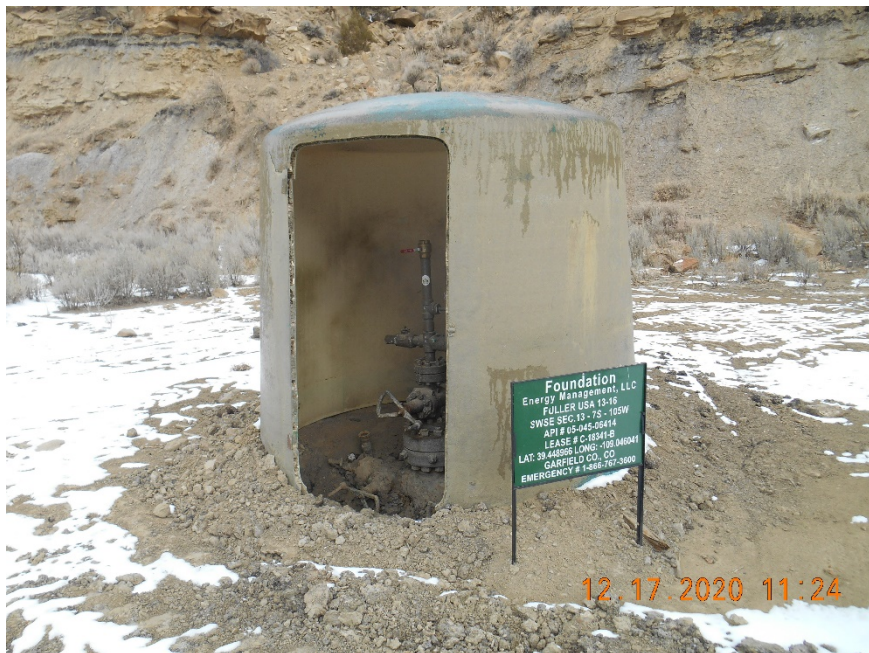
Wellhead inside housing with sign
