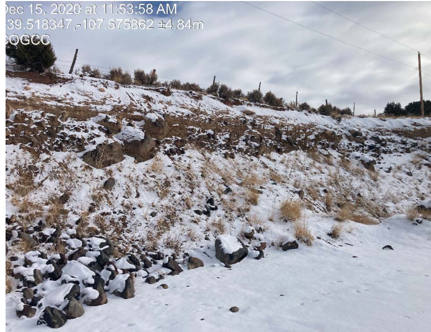
Cut slope requires stabilization
