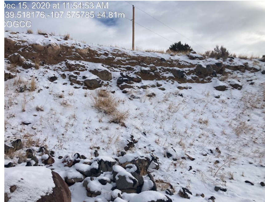
Cut slope requires stabilization
