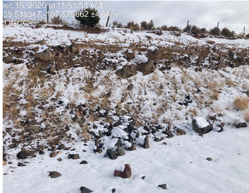
Cut slope requires stabilization
