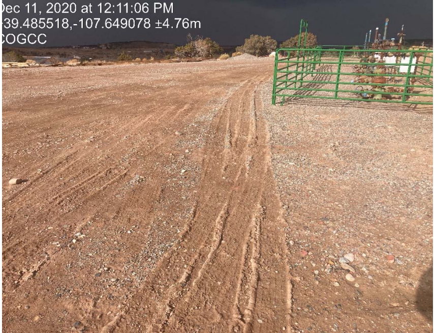
Lack of stabilization
