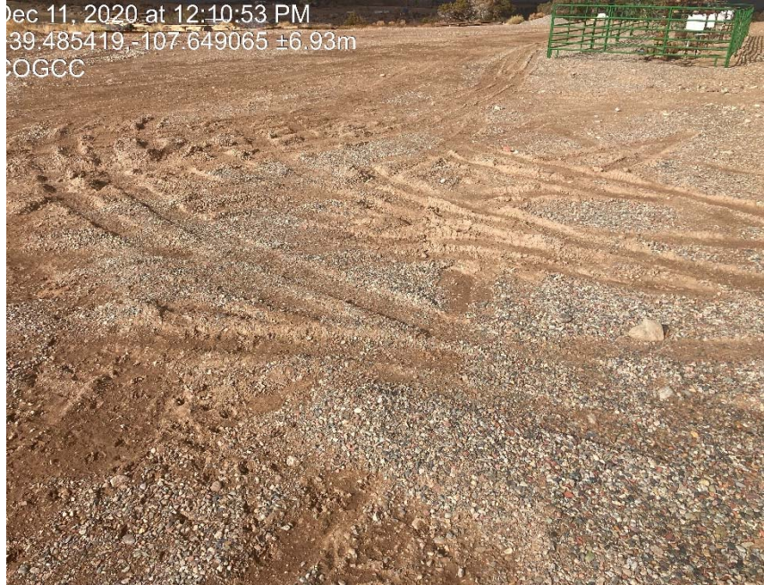
Lack of stabilization
