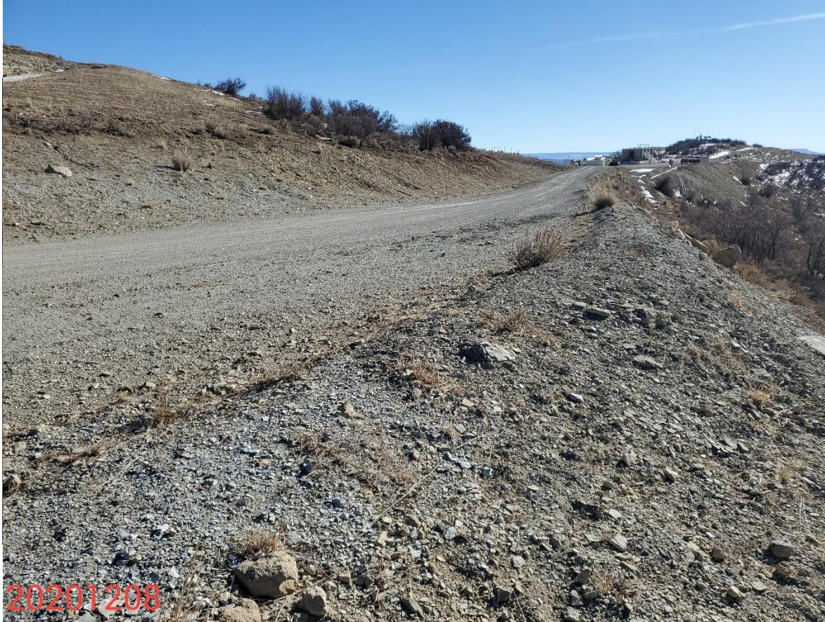
Photo 10: Photo taken from the southwest corner of the Cascade Creek 697-04D location. Photo shows additional access road leading to the CC 0604-1 Pad. This is additional disturbance that does not comport with Rule 1002.e
