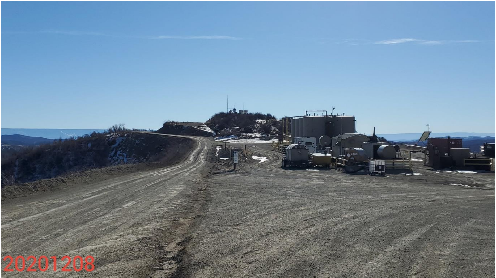
Photo 9: Photo taken from the north end of the CC 0604-1 Pad Location, facing south. There are currently 2 access roads, and 4 access points (on the northwest, northeast, southwest and southeast) to the CC 0604-1 Pad . Photo shows eastern access road
