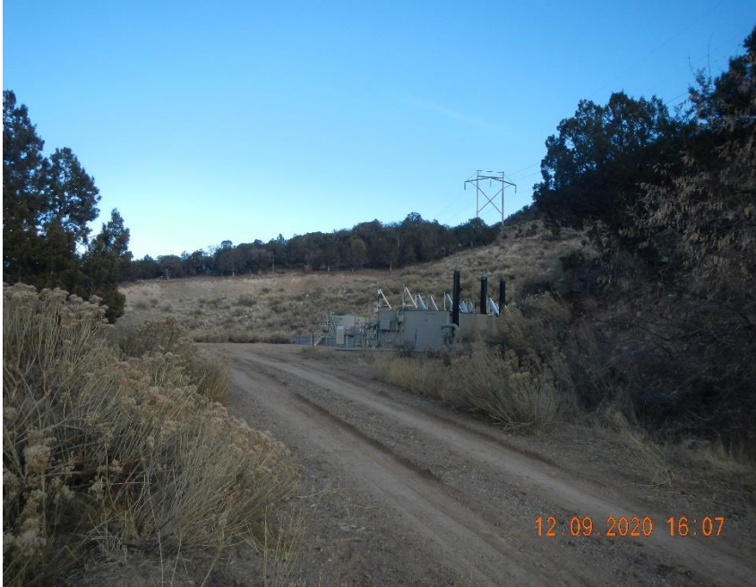
Ruts on access road.
