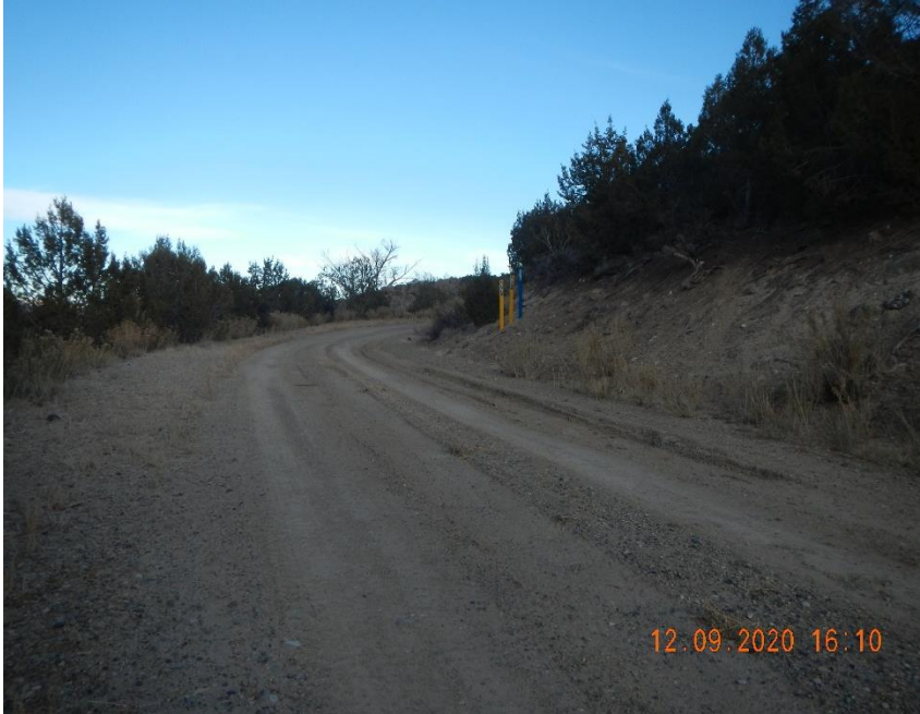
Ruts on access road.
