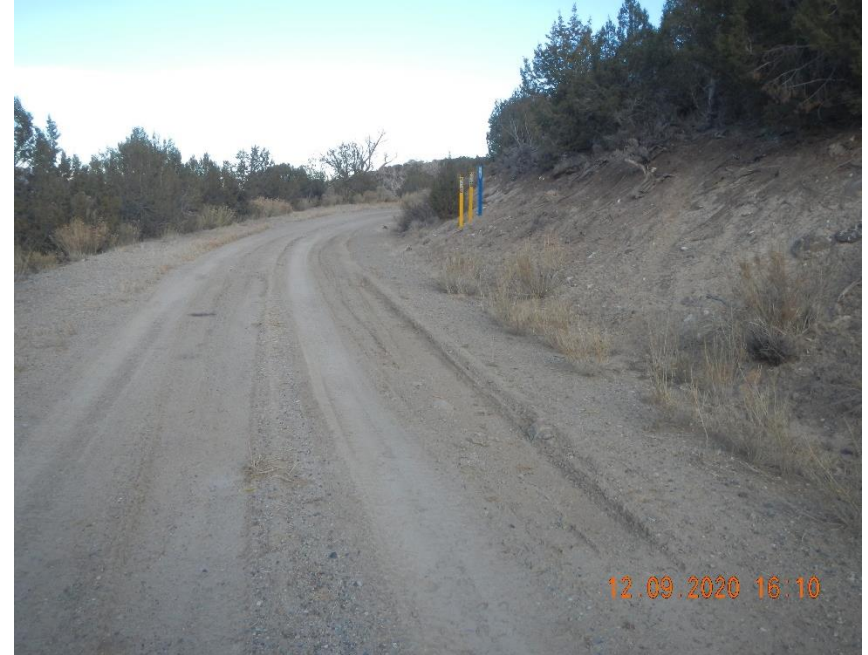
Ruts on access road.
