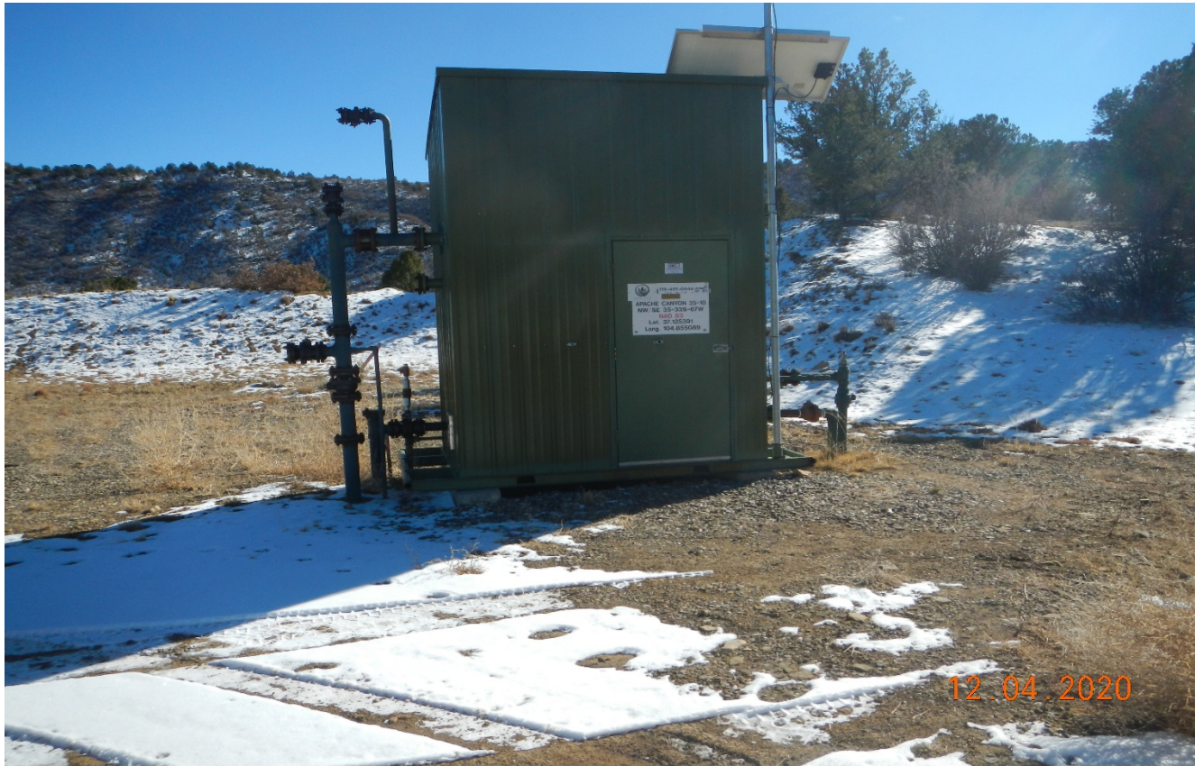
Photo 3. Well sign posted at meter shed.
