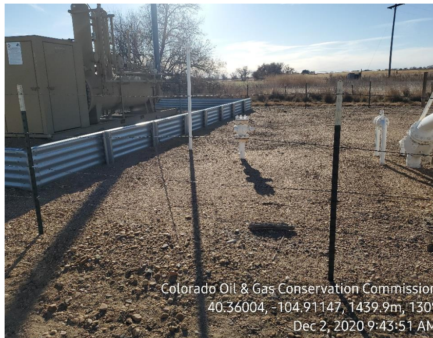
Photo 3: Risers needed to operate facility
