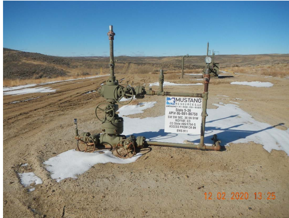
Photo 1. Overview of location taken facing north. No bradenhead access. Previous operator on signs.
