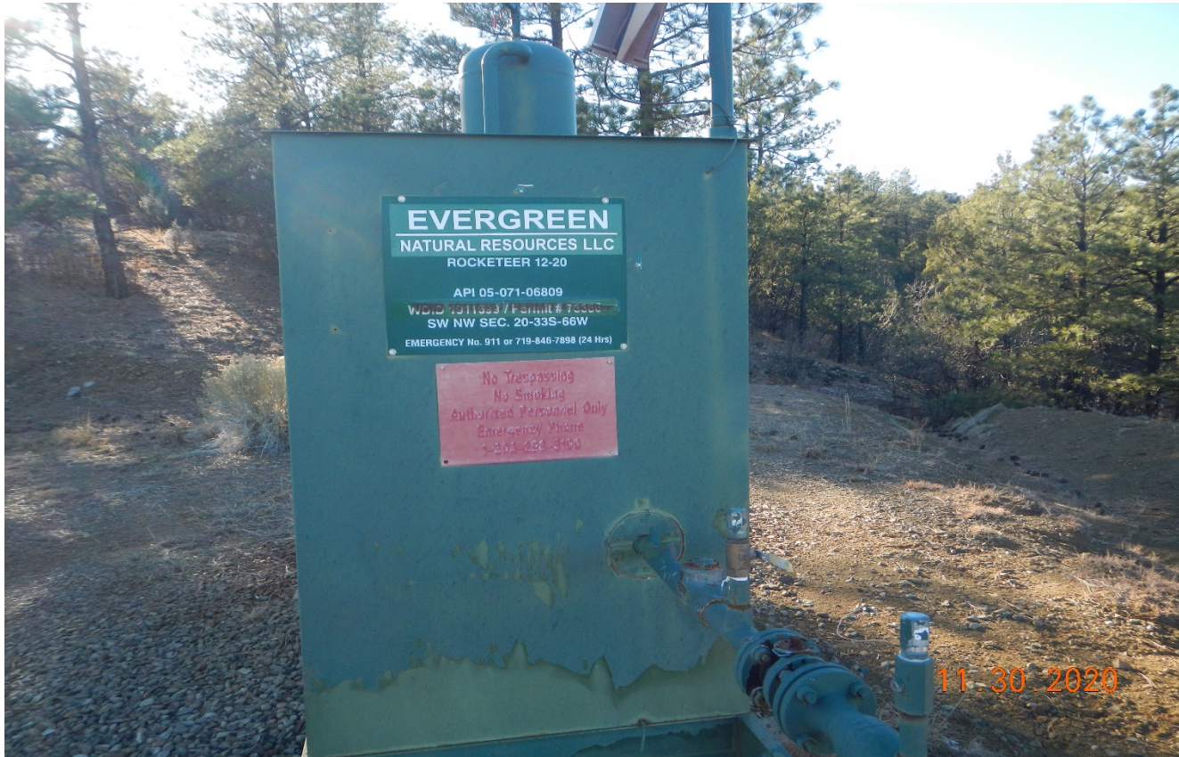
Photo 1. Well sign posted at meter shed.
