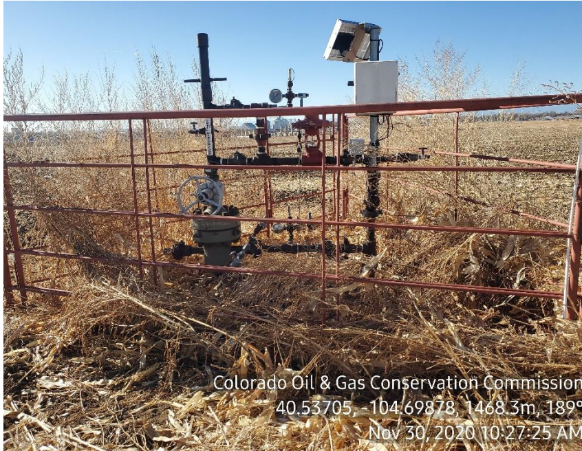
Photo 1: Wellhead; No sign displayed
