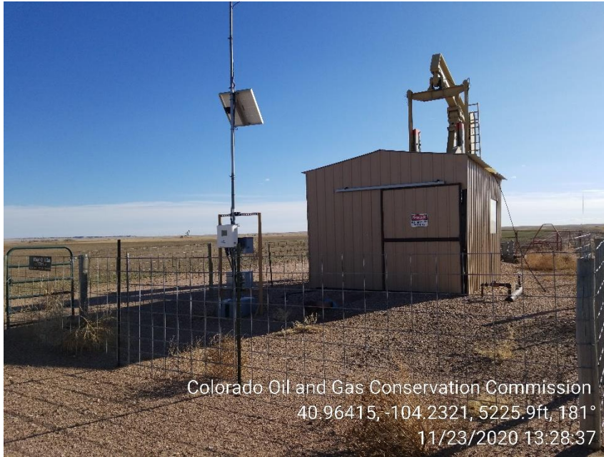
Photo 3 – Pumping Unit, weeds
