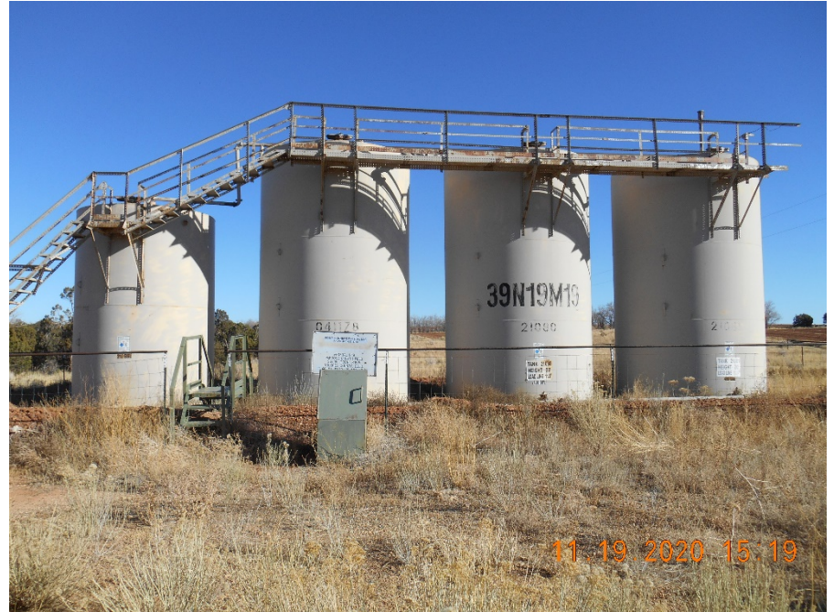
Tank Battery with earth berms.
